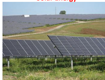
11 MW Serpa solar power plant in Portugal
