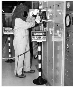
Art Wise in protective clothing and gear as he inserts a starter bucket into a Motor Control Center.
