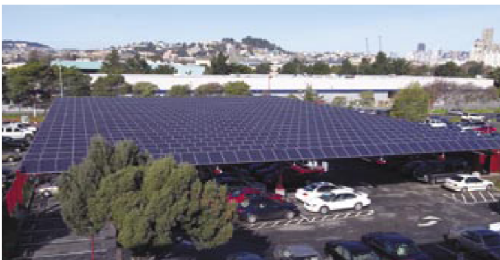
The solar photovoltaic system at the San Francisco P&DC is mounted on a parking canopy that tracks the movement of the sun.
